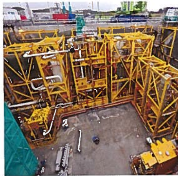
Ormen Lange pilot compressor train in seawater basin prior to flooding
