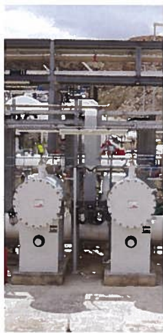
Filter/water separators at an airport fuel storage facility
